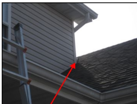
Recommend extending 2nd floor gutter downspout down to lower gutter.
