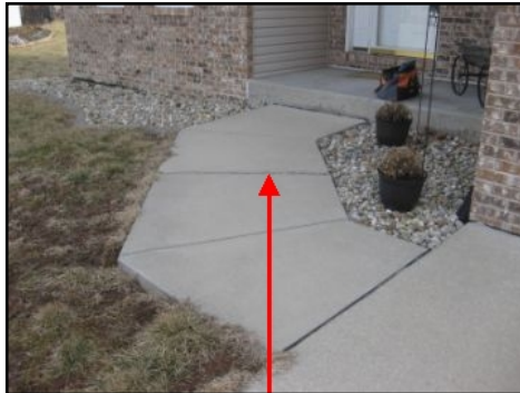
Trip hazards in walkway, exercise caution.
