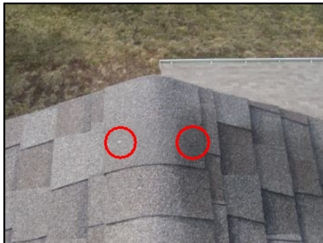
Exposed nail holes should be sealed.
