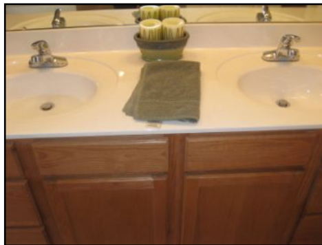
Left sink drains very slow.
