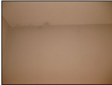
Ceiling areas have some stains.
