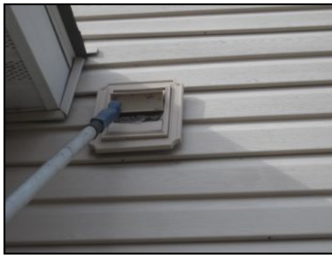
Exterior dryer vent needs cleaned out.
