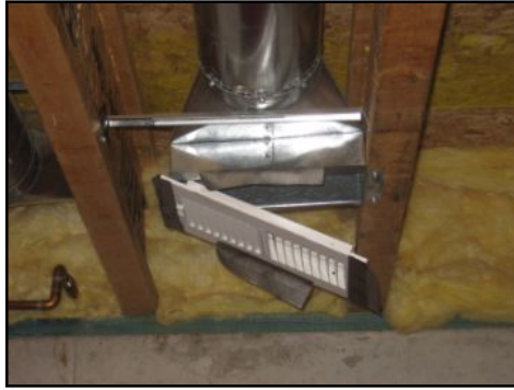
Loose register in basement needs secured.
