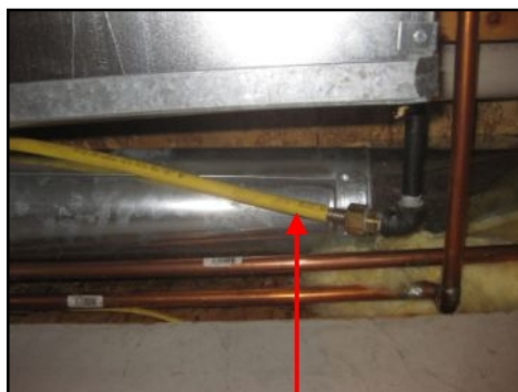
The csst gas line needs to be bonded to a suitable ground.
