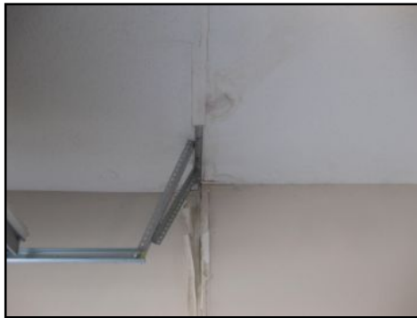
Past water leak and minor damage noted on north ceiling and wall.
